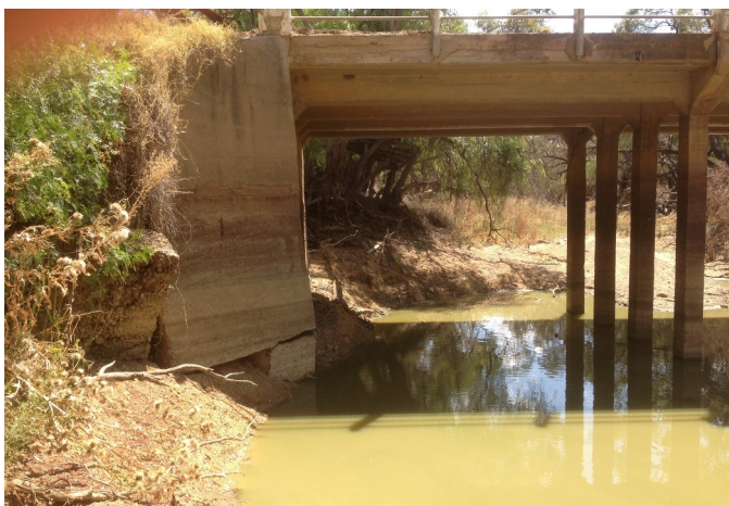
Culgoa bridge was extensively damaged during the flood
